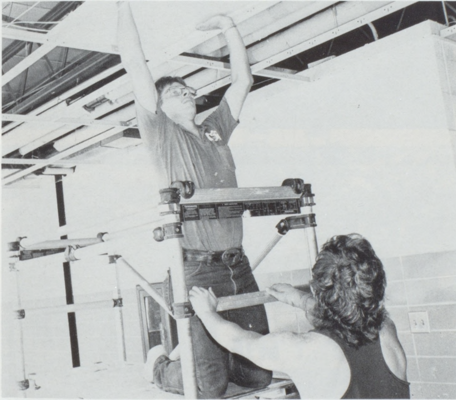
Workers remove asbestos from the ceilings of CHS during the summer of 1989. The asbestos removal is just one of the improvements the high school underwent. -photo Citizen Observer
