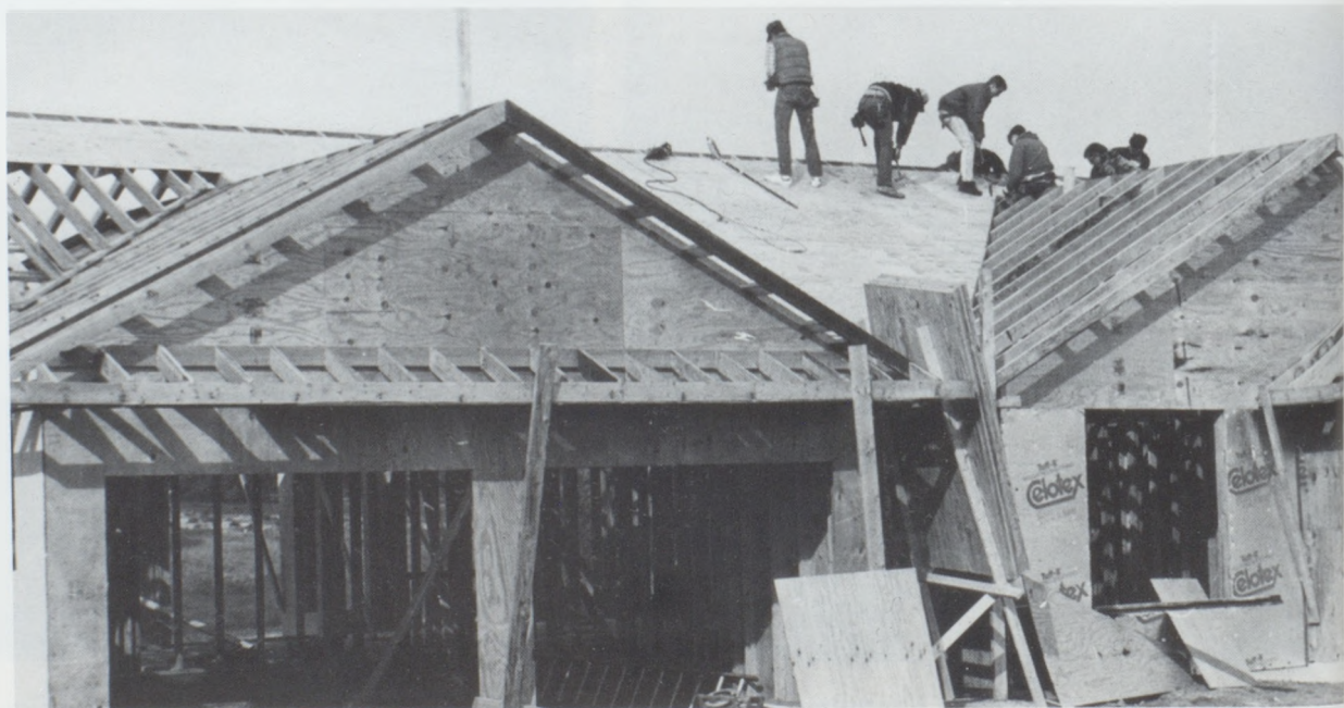
Morning Carpentry class works busily to finish the roof before the colder weather comes.
