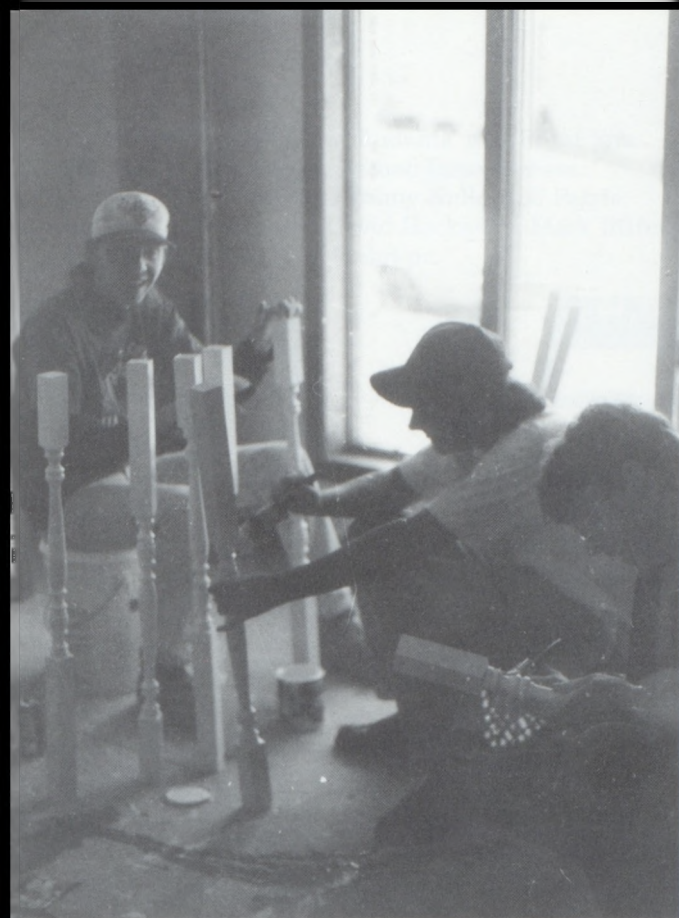
M att Berry, Jason Hahn and Chuck Willits paint the spindles to be put in the stairway.
