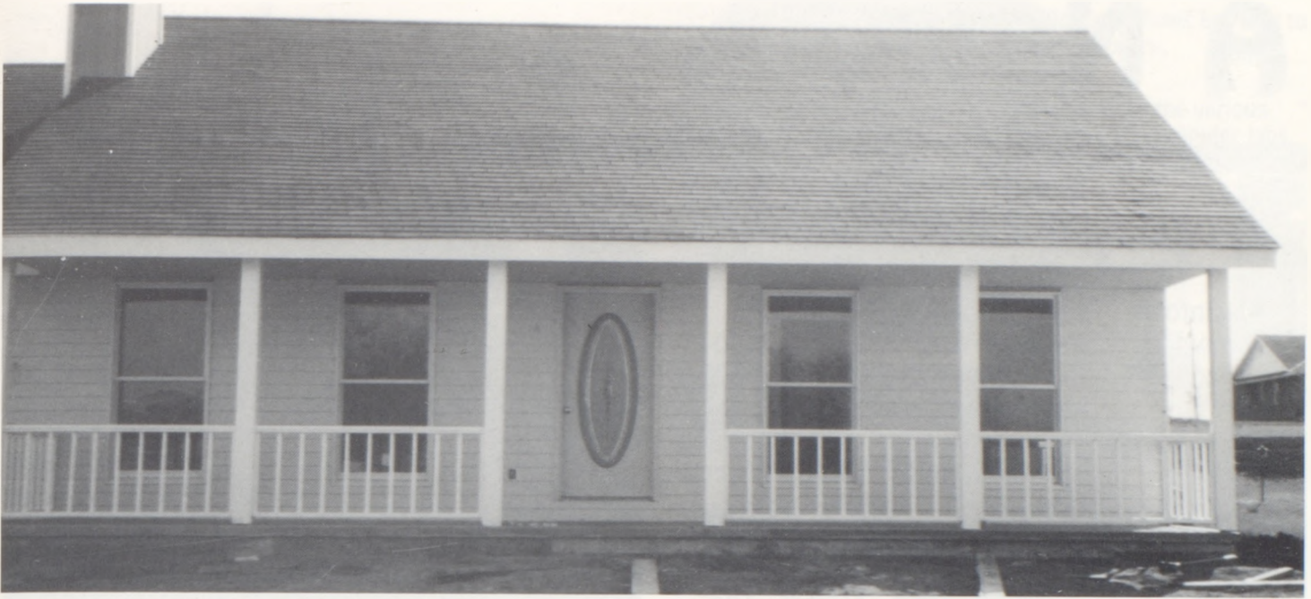
The carpentry house being put into the works by CHS carpentry and interior design students.
