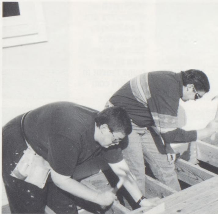
Brian Burnett and Dallas Fox fit into a tight squeeze while adding the boards to the deck.
