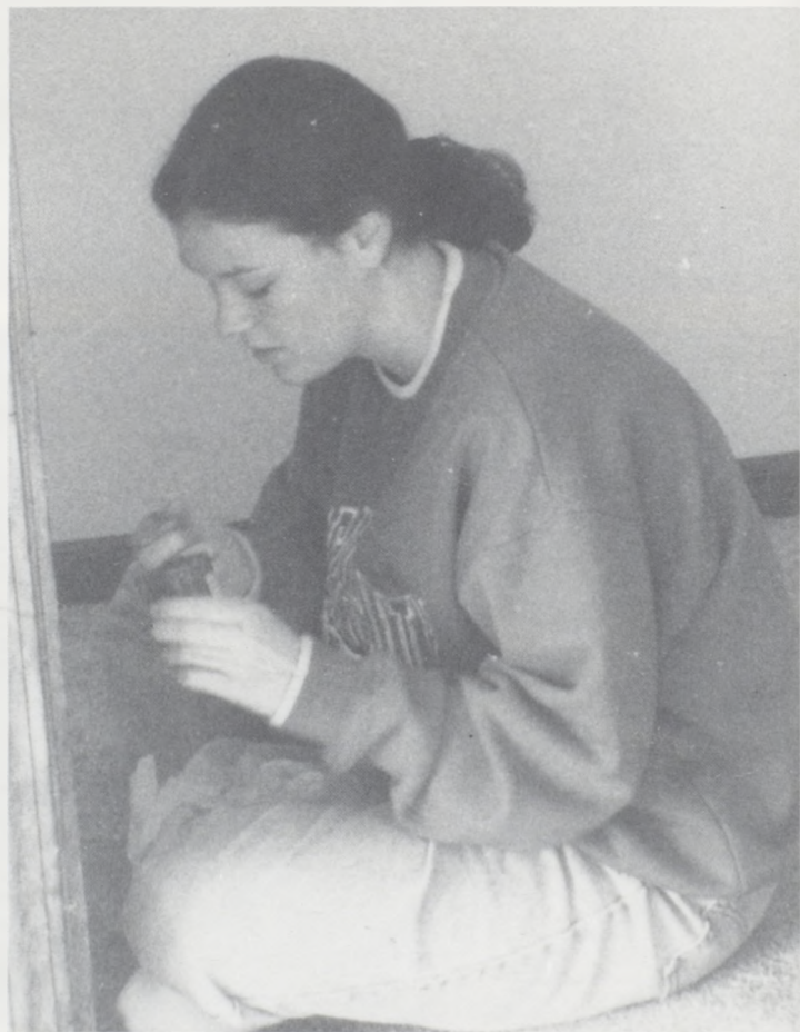
Lori Parks is concentrating hard on filling in the nail holes, while sitting on the brand new carpet.
