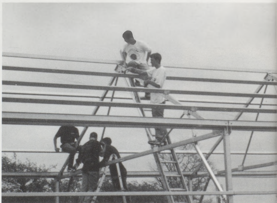
It's about to storm as Ben Miller and Justin Curtis sit on top the greenhouse and try to fit in some last minute work.
