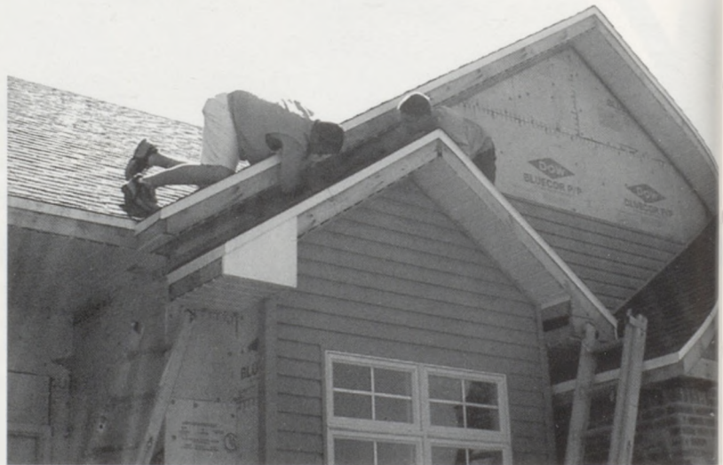
M aking sure the roof dosen't blow away is Luke Schlorff and Eric Brownlee.
