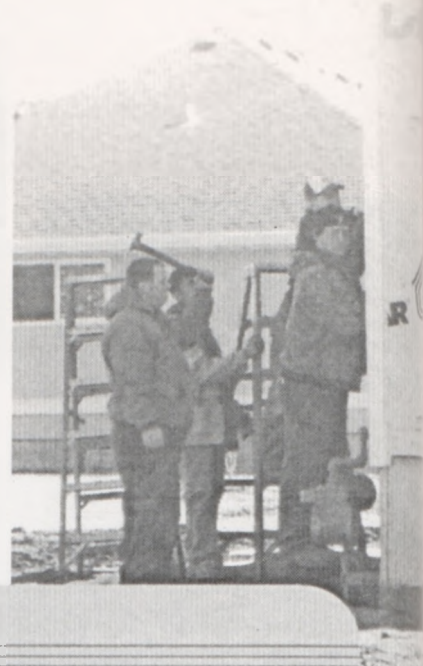
1 Working together, the gold day carpentry class begins putting up the siding to complete the outside touches of the house.
