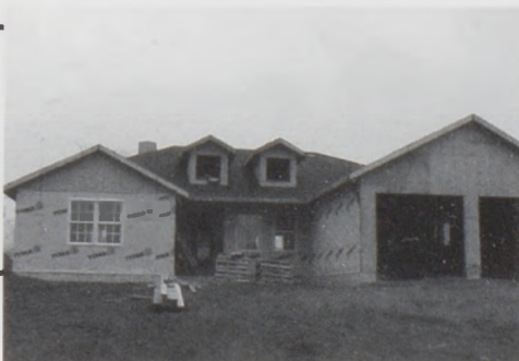
Left: Carpentry house lookin pretty good just in time for the cold weather!
