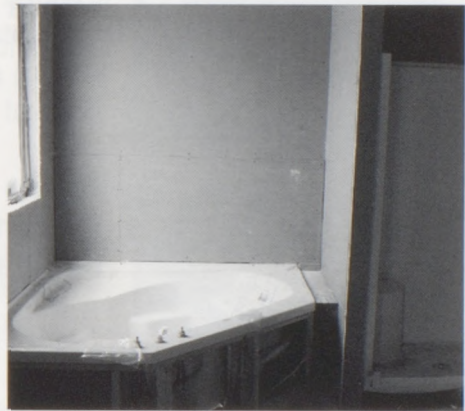
The corner whirlpool tub is roughed in and ready for the detail work.
