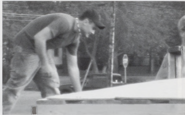
Chad Utt prepares to move a sheet of plywood into the house.
